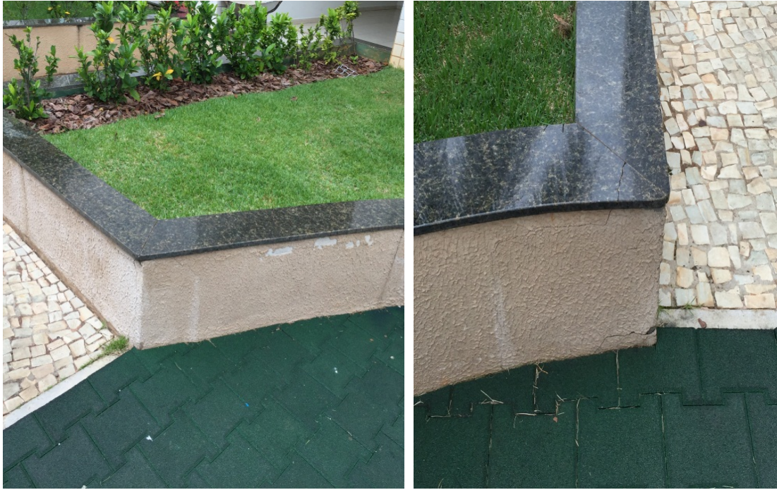
Muretas com pintura descascando no playground
